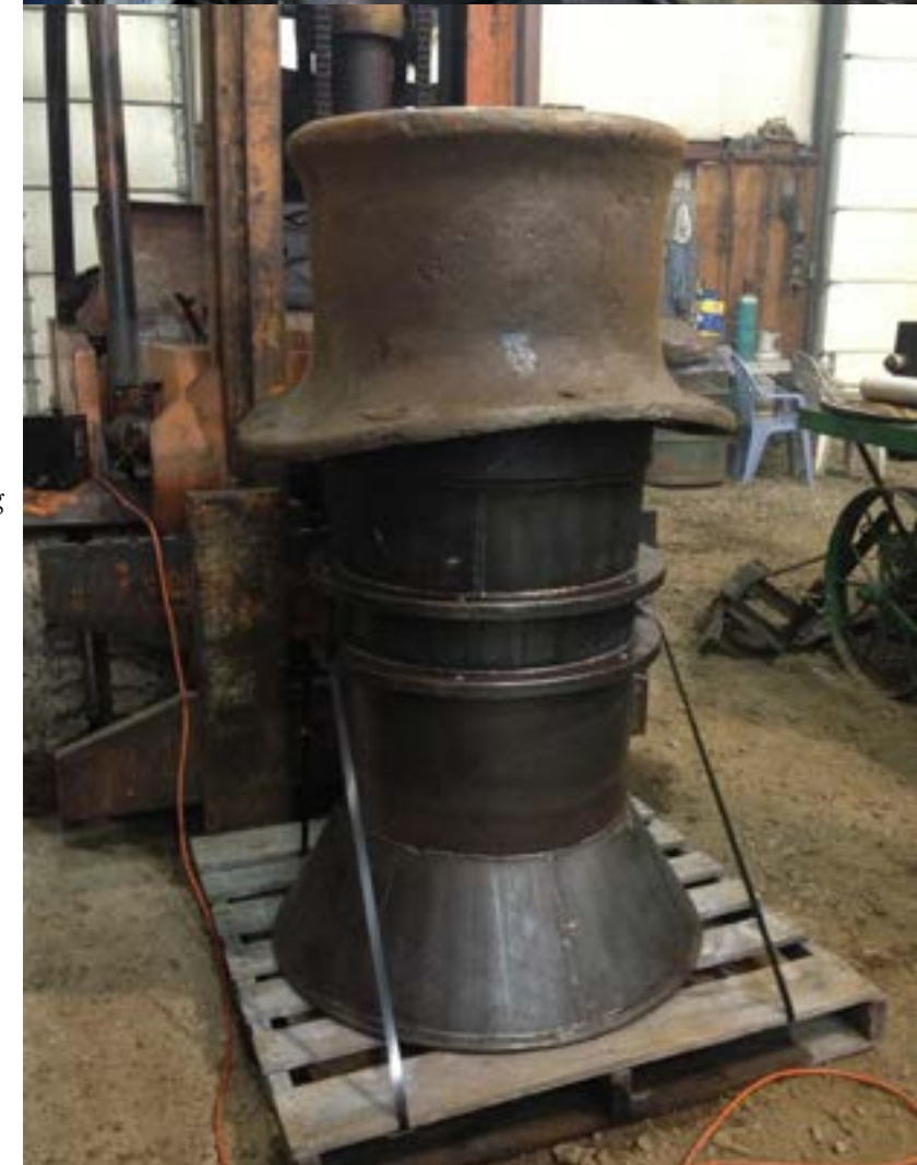
George Kester (above, left) and Brad Taylor (above, right) team up to prepare the installation of a new smokestack and petticoat structure to replace the 1944 original. The new smokestack and other parts were formed by Charles Overley Fabrication in St. Marys, Ohio.
